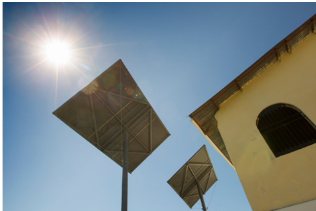
Solar panels power a computer lab at the Thomas Food Project in Thomas, Haiti. A UMNS photo by Mike DuBose
